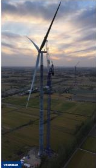
INNOVATIVE WTG INSTALLATION FROM YONGMAC Pioneering Yongmac tower crane (model SET2) set records (over all in height) at 182m.
