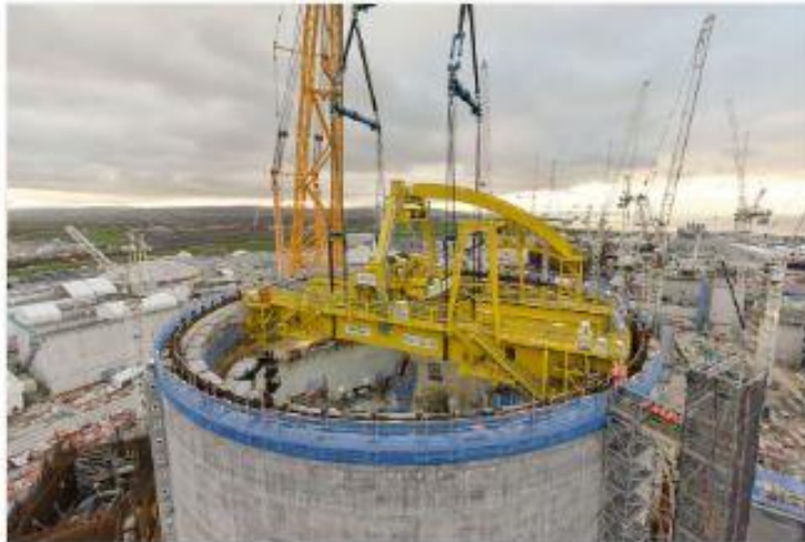
Sarens' Big Carl places the polar crane which rotates inside the top of the reactor building. Photo: EDF Energy
