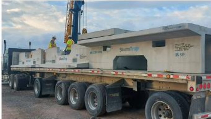
SARENS — Sarens has participated in the installation of a storm trap on the North Service Road in Burlington, Ont., where it has been able to provide its crane to the construction team for the lifting and placement of each of the modules.
