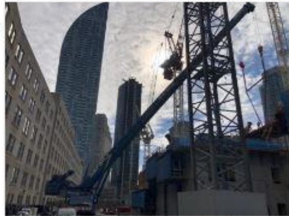
Sarens, global heavy lifting, engineered transports, and crane rental services firm, assisted SuperMetal in the construction of the Union Station overbuild in downtown Toronto. Photo courtesy Sarens.
