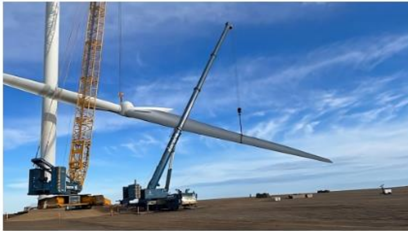
A Demag crawler crane and Liebherr all-terrain crane were used to handle heavy turbine life in Assiniboia, Saskatchewan. (Sarens)
