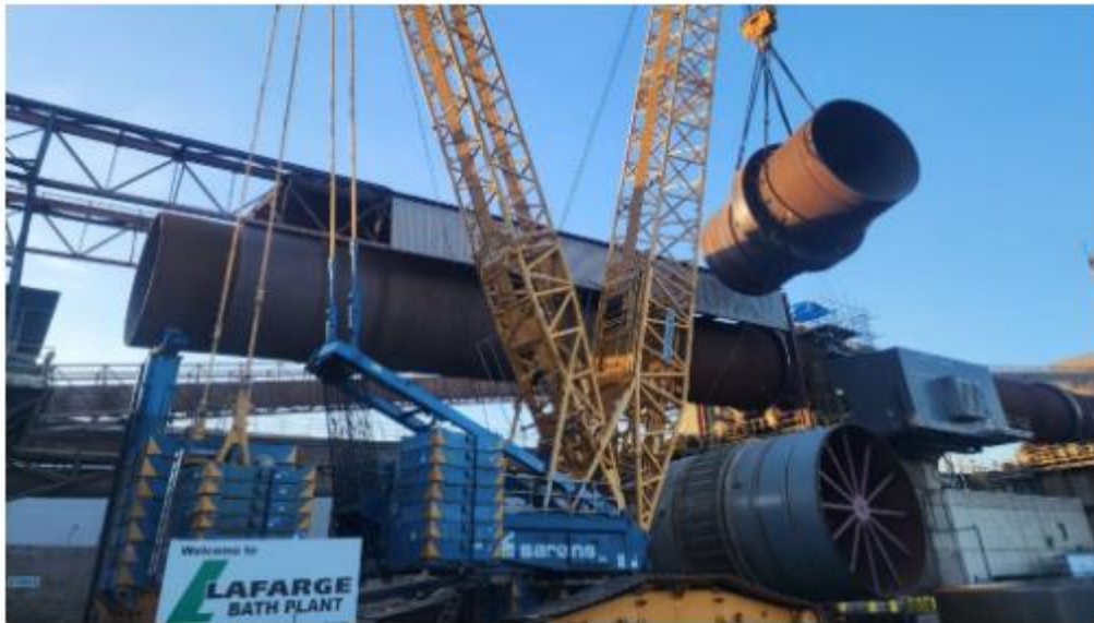
Sarens used a Liebherr LR1600 crawler crane for the kiln dryer replacement project. (Sarens)
