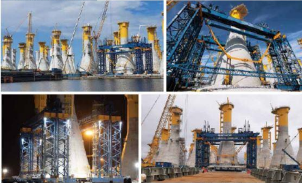
Each of the 71 concrete structures has a 31m diameter base, is 48-50m high and weighs 4,800 tonnes
