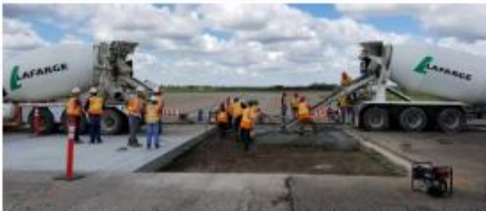
The kiln dryer replacement project is part of Lafarge's plan to reduce its carbon footprint through a new sustainable policy.
