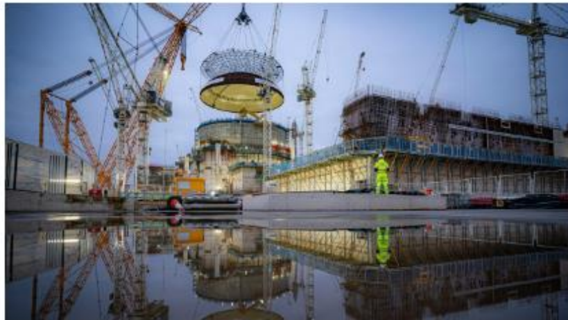
"Big Carl", thought to be the world's largest crane, lifts the 154ft-wide steel dome into place early on Friday morning
