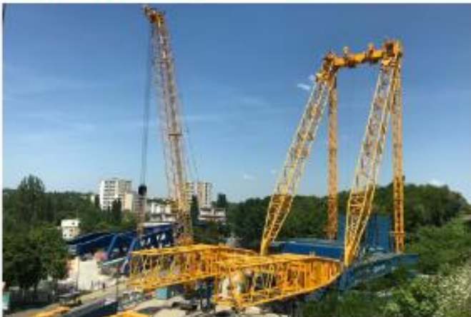
The base of the SGC90 crane is assembled on the ground before being moved to the location for the new bridges. © SARENS
