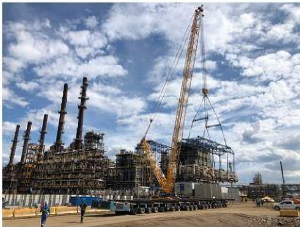
Sarens understands the importance of maintaining a stable investment in technological innovation in the construction of new oil sands processing infrastructures and in the gradual renovation of existing ones (photo: Sarens)
