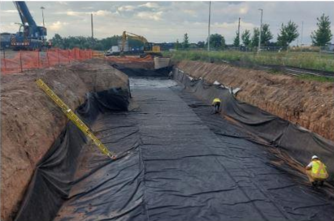
Sarens recently deployed a Liebherr LTM 1070 mobile crane to assist Valentine Underground Services complete a storm trap installation in Burlington, Ontario.
