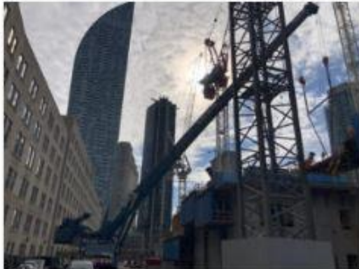
Sarens, global heavy lifting, engineered transports, and crane rental services firm, assisted SuperMetal in the construction of the Union Station overbuild in downtown Toronto. Photo courtesy Sarens.
