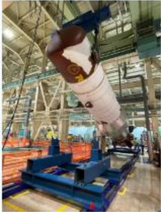
SARENS SETS INDUSTRY RECORD REPLACING TWO HEATERS AT U.S. NUCLEAR STATION Sarens installed 2x 100-ton heater heaters in an plant at Cherokee Nuclear Station in South Carolina, USA.
