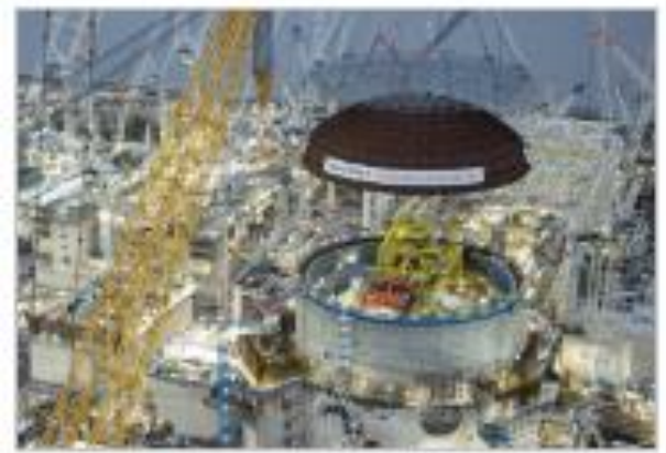
Teams waited for the perfect wind conditions to lower the dome into place.
