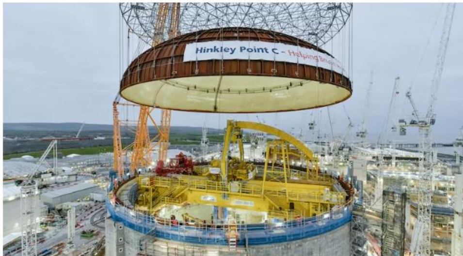
The dome being lifted into place by the gigantic crane, which has 12 engines and can lift up to 5,000 tonnes – equivalent to 10 jumbo jets. Courtesy EDF
