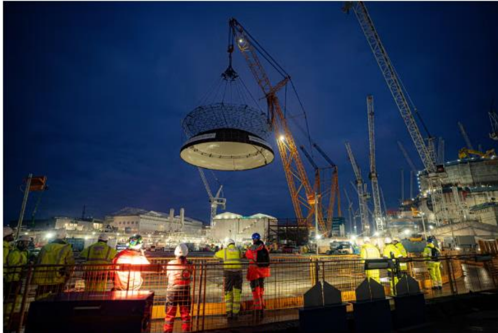
Engineering teams use the world's largest crane – Rio Carl – to lift a 245-tonne steel dome onto Hinkley Point C's first reactor building (Ben Birchall/PA) /PA
