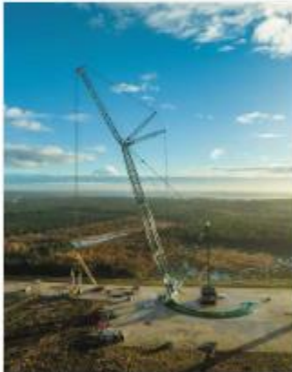
BMS' new 3,000 tonne capacity ring crane. (Photo: BMS)
