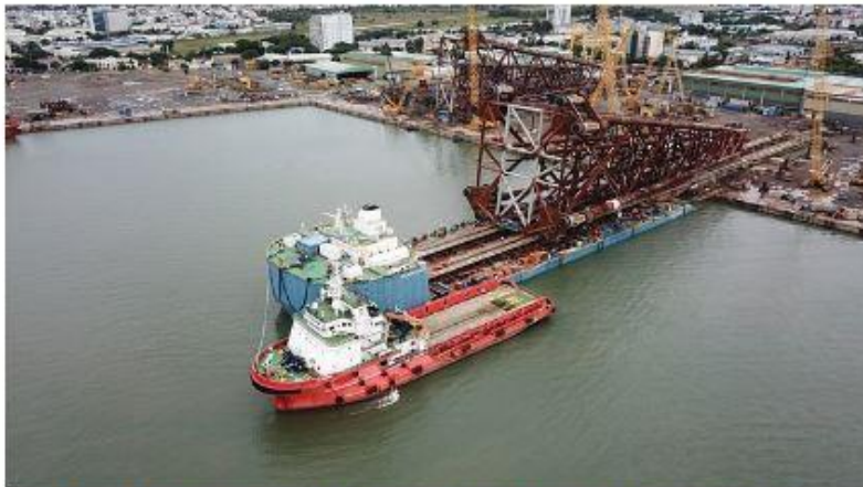
Sarens has been in charge of loading two of the project's jackets out, the ZWP12 and ZWP15, weighing approximately 5,000 tons each, on behalf of the Vietsovpetro joint venture (photo: Sarens)
