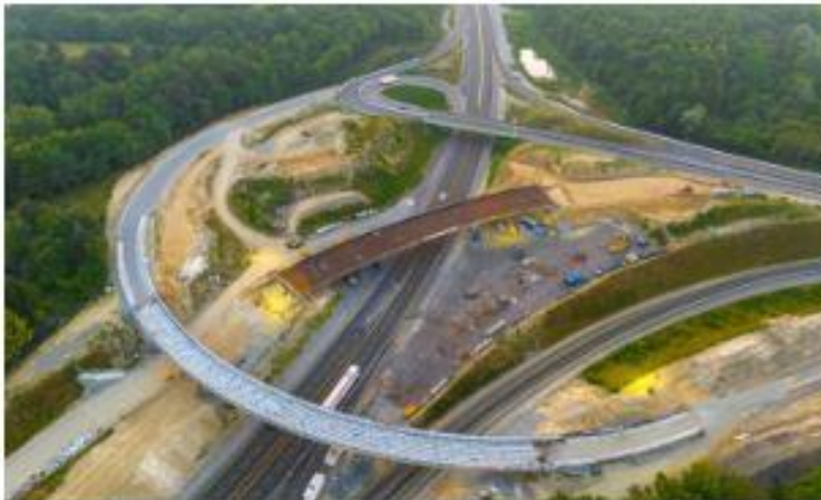
Because the job site was located along the A11 autoroute, there was limited space and access for vehicles and equipment. (Image courtesy Sarens)
