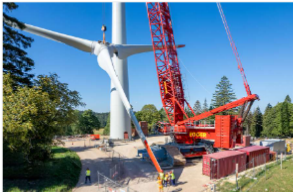
Emil Egger's Liebherr LR 11000 begins to hoist a wind turbine rotor star. Photo: Liebherr
