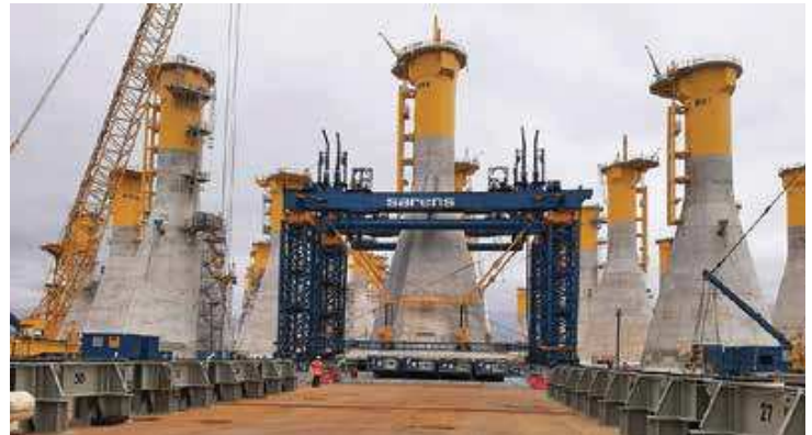
Each of the 71 concrete structures has a 31m diameter base, is 48-50m high and weighs 4,800 tonnes
