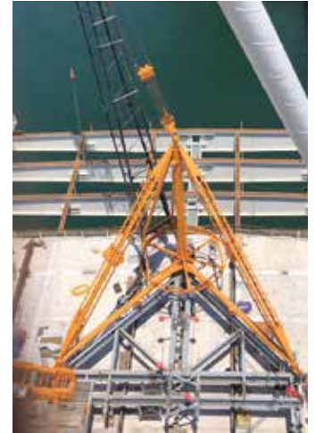
Each pair of derricks face and move away from the towers in opposite directions
