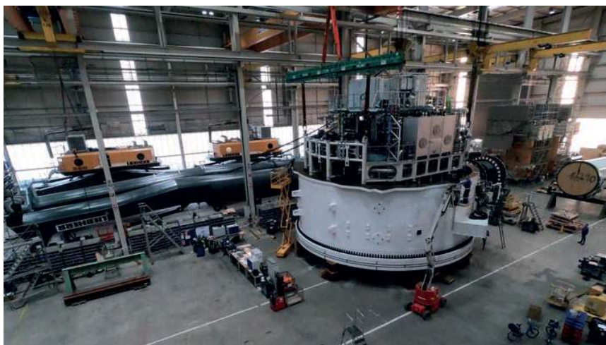
A landmark moment: the lower slewing unit of the Liebherr HLC 150000-3000 is now complete
