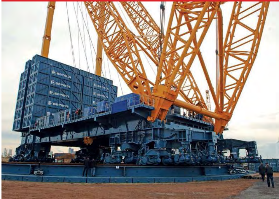
Just over 5,000 tonnes of counterweight accounts for more than half of its 9,000 tonnes total weight
