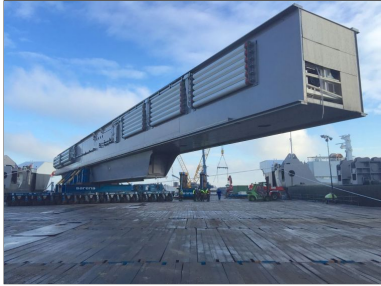
Additionally, Sarens was contracted by tenants in 2014 for the jacking - loadout and transfer of the vessel's 4,200 tonne, 150 m long and 65 m wide stinger. The first step of the operation was the jacking up of the stinger using Sarens' C15000 jacking system, which allowed tenants to finalize the construction. The completed stinger was subsequently transferred from the construction location in Wassagen, the Netherlands, to Alsea's purpose-built stinger barge, Bumblebee.
