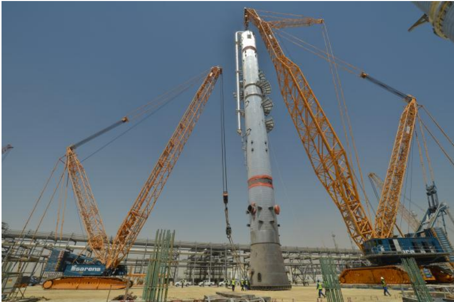
CC 8800-1 Boom Booster (right) lifting a column at Sadara Project, Saudi Arabia (photo: Grzegorz Dajer)
