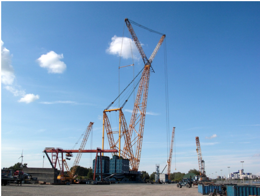
SGC-120 in Ghent, Belgium
