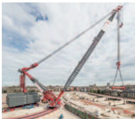
ALE has finished using its AL.SK190 crane at Earls Court in London, UK, where it says it lifted a beam weighing 1,500 tonnes - the largest single lift undertaken in UK history
