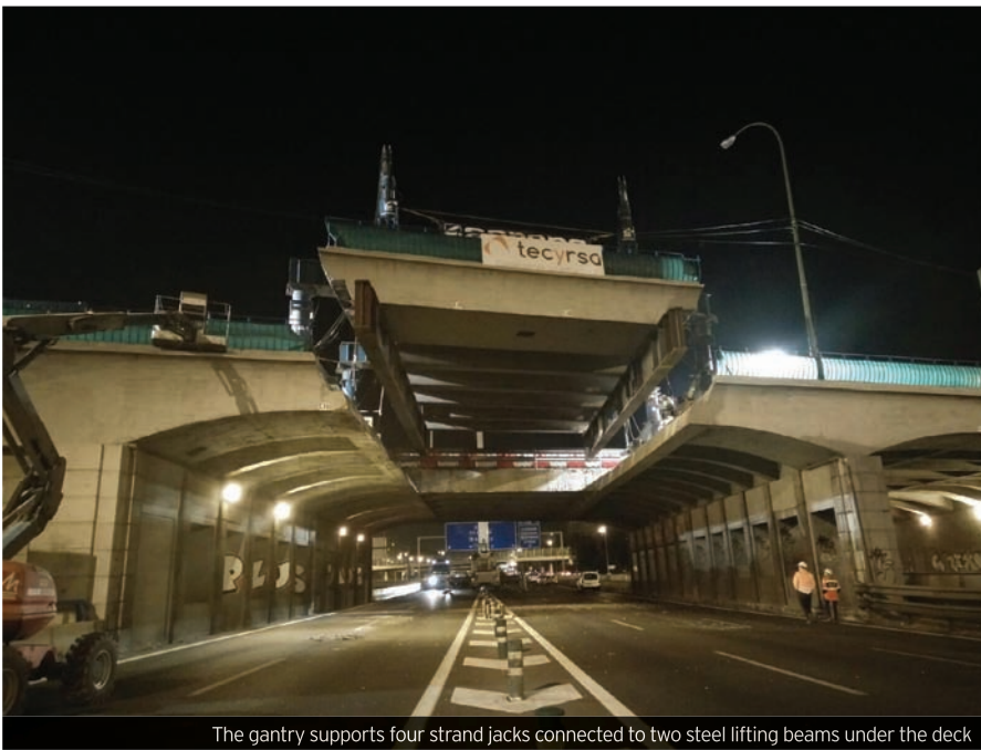
The gantry supports four strand jacks connected to two steel lifting beams under the deck
