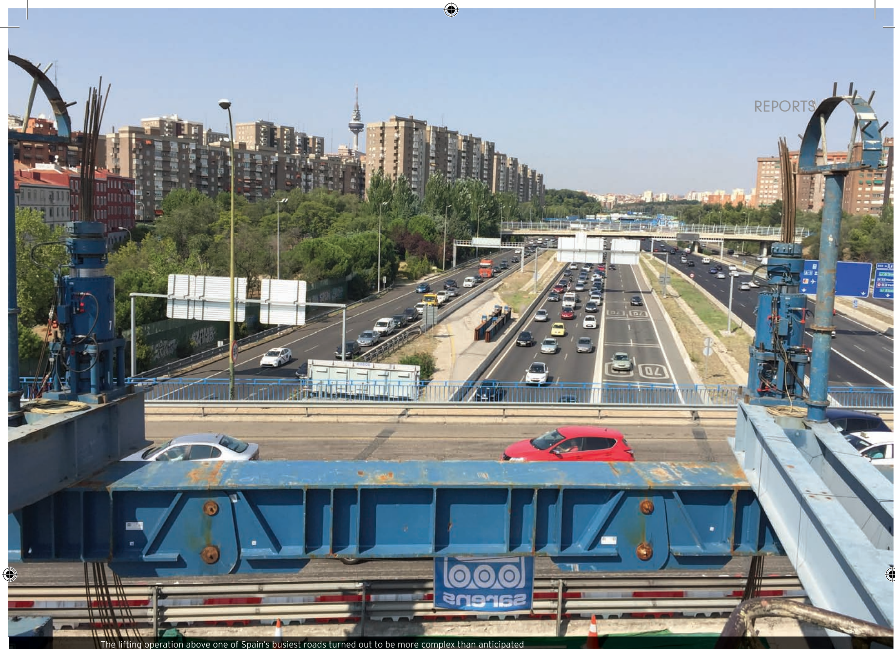
The lifting operation above one of Spain's busiest roads turned out to be more complex than anticipated
