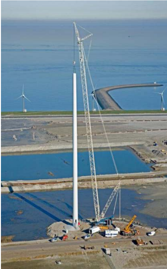
Vestas Benelux Eemshaven V90 (3MW) / 100m
