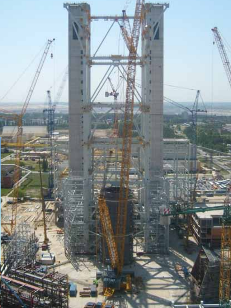
Belchatow (POL) Building Concept based on: CC8800/1, 2xCC2800/1 2 x Portal tower cranes Peiner VM1300
