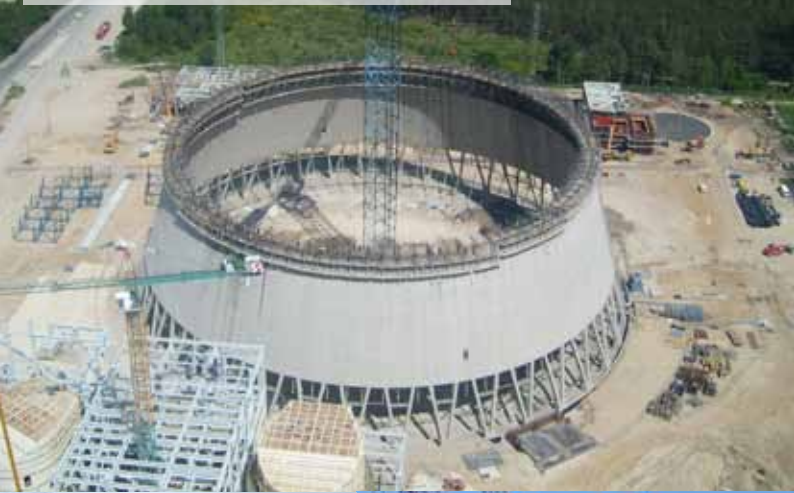
Belchatow (POL) : Cooling tower construction Heavy Lift tower crane Free standing up to 100m
